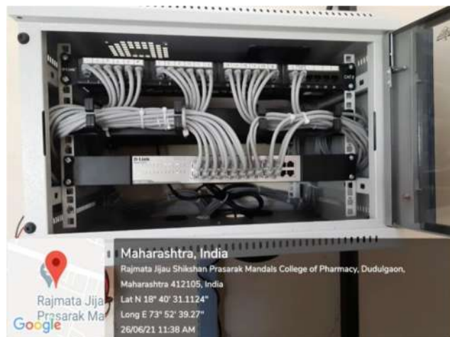
Cable network of internet in Computer Lab
