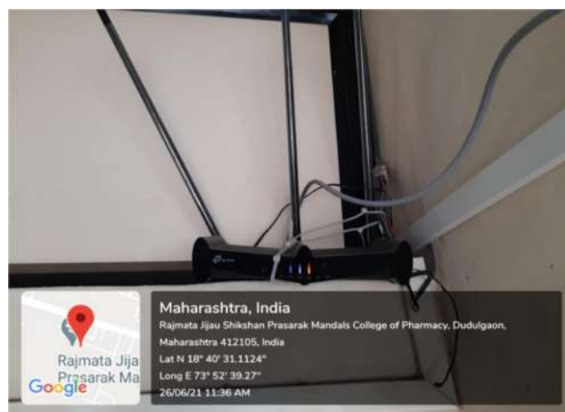
Connection of cable to router in office
