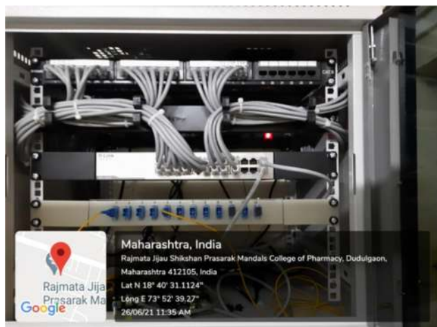
Cable network of internet in office
